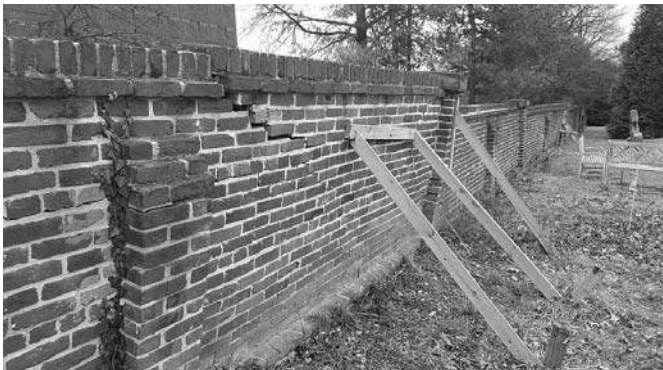
Leaning wall prior to demolition and reconstruction.
